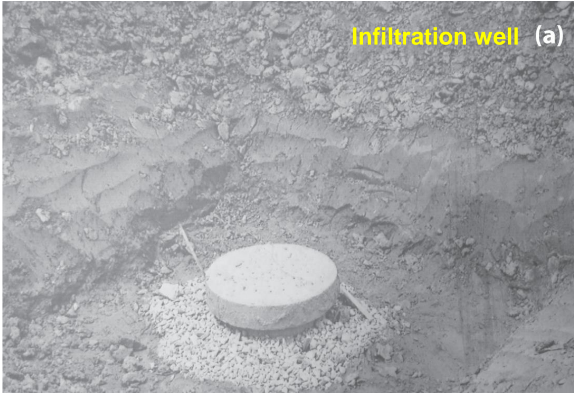
(a) Drilled infiltration well of ~ 20 m deep at river bed. The well is capped with a slotted concrete cover and sits in a catch pit which has not yet been filled with coarse materials
