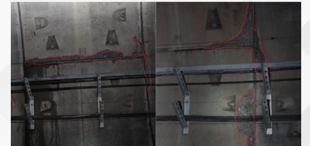
Intelligent spalling detection
